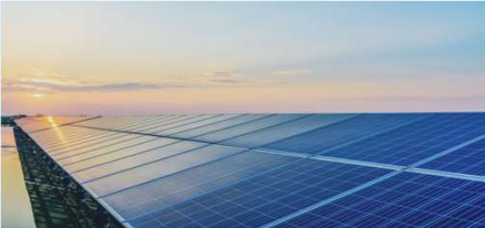
Solar power sourcing projects are initiated at Rudrapur, Ambernath and Khopoli plants
